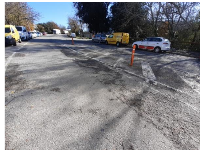
Fissures, trencaments, desprendiments i deformacions.
