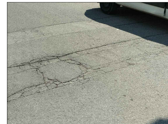
8. Tram 1 C. Chopin. Fissures.
